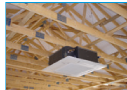
Air conditioning units
